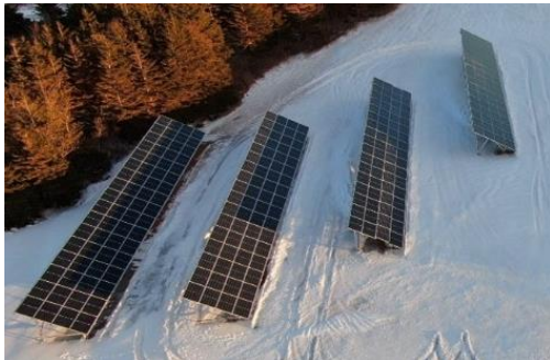
Figure 1. Aerial view of WEICan's PV array
