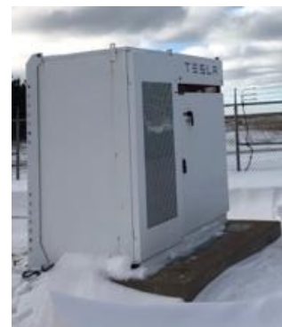
Figure 2. WEICan's battery energy storage system (BESS) ,
