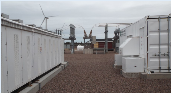
Fig 2. Battery Energy Storage System at the Wind R&D Park (the substation and a turbine are in the background)
