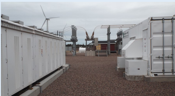
Fig 2. Battery Energy Storage System at the Wind R&D Park (the substation and a turbine are in the background)
